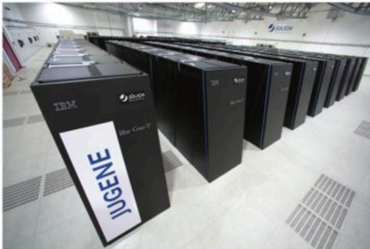
FIGURE A-4: Supercomputer
